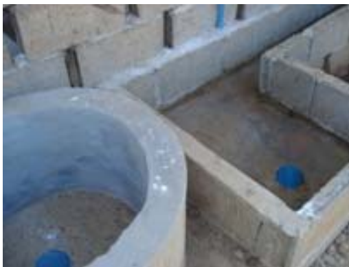
Photo-4.1: Inlet tanks
