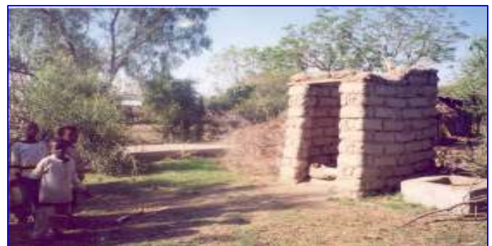
Connected toilet in need of maintenance
