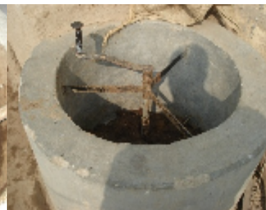
Photo 4.3: Inlet of GGC Plant (small)
