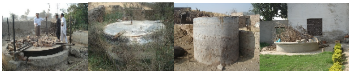
Photo 4.11: Different Conditions of Non-operational Biogas Plants
