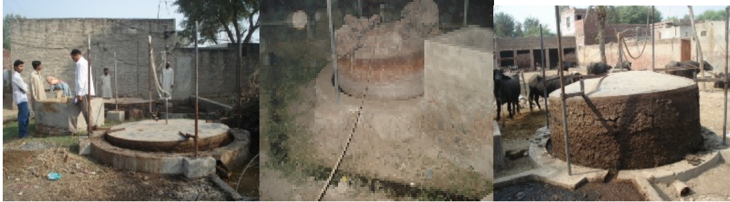
Photo 4.9: Improper system of pipe lines to convey biogas to point of application
