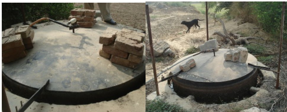
Photo 4.4: Load added on top of drum to build pressure. Drum is tied with the poles.
