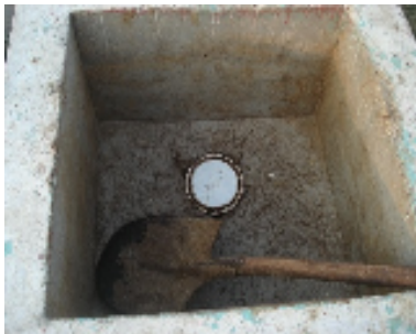
Photo 4.1: Inlet of Floating Drum Plant
