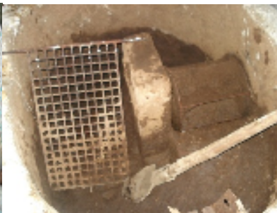
Photo 4.2: Inlet of GGC Plant (big)
