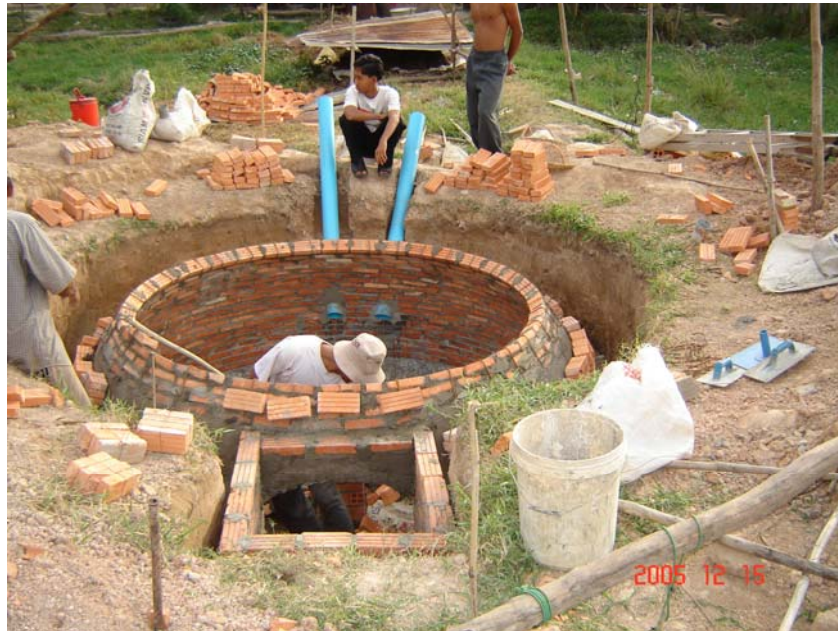
A 6 m 3 Farmers Fried biodigester under construction at the Royal University of Agriculture in Phnom Penh
