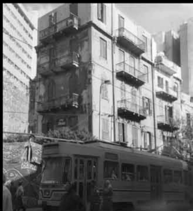
The neglected façades of an apartment building, on which an extra floor was built. The continual vibrations from the passing tram and heavy traffic have contributed to the deterioration of such buildings.
