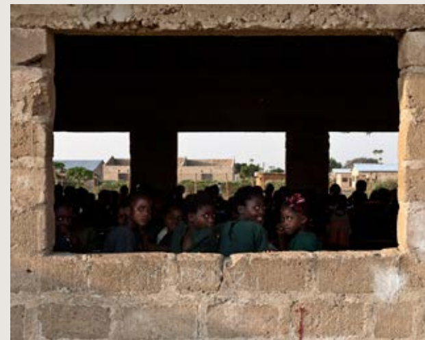
Pupils at Nakambala Basic School, next to the Zambia Sugar estate, in their unfinished classroom.
